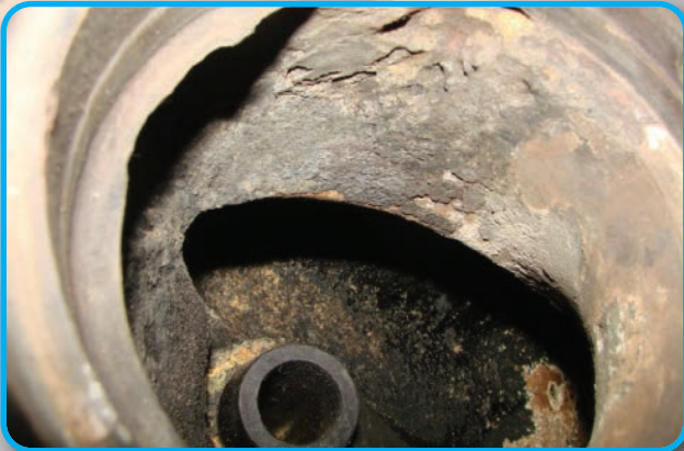
Exhaust Gas outlet port deep corrosion
