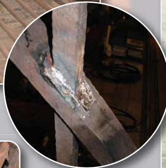
Joints loosened in the collision were refilled with lead, the method used in the gates original construction.
