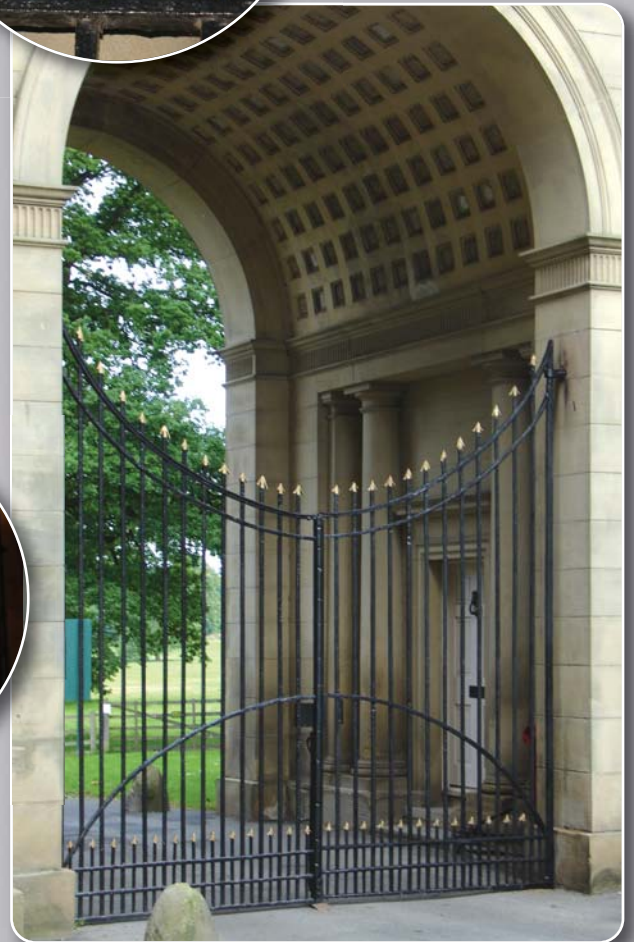
The refurbished gates. In position and resplendent in a new coat of paint.
