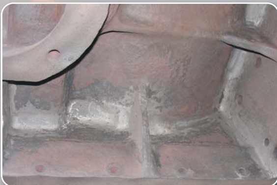
Close-up of complete block after sand blasting showing additional re-enforcement giving extra strength to the repaired area before prima painting.
